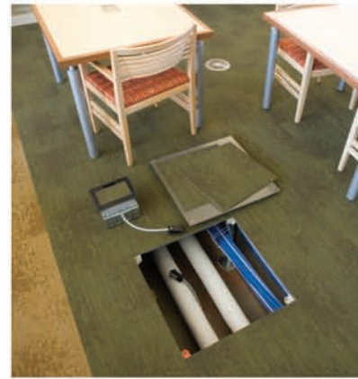
The Library's innovative raised floor allows for underfloor air circulation, which maximizes the efficiency of heating and cooling, saving energy and taxpayer dollars.
