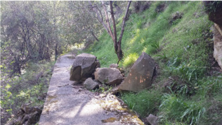
Localized rockslides are common within the steeper sections of the Canyon; here rocks fell atop the Sunol Aqueduct east of the Farwell Bridge
