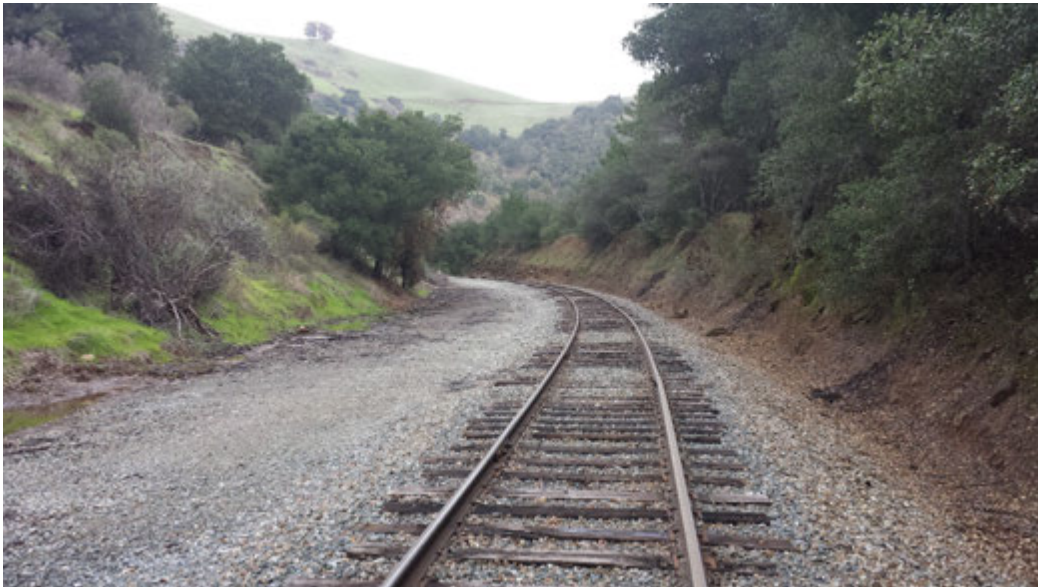
Along segments of the Niles Canyon Railway, there is adequate area to place a trail.
