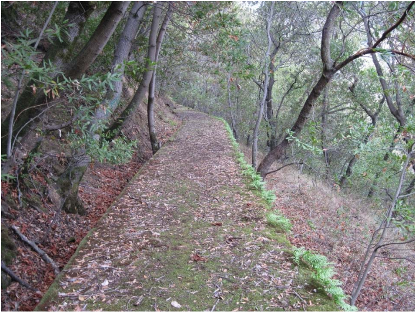
The deactivated Sunol Aqueduct runs above ground providing an accessible path through portions of the Canyon. The aqueduct is popular destination for locals who now know it as the "secret sidewalk."
