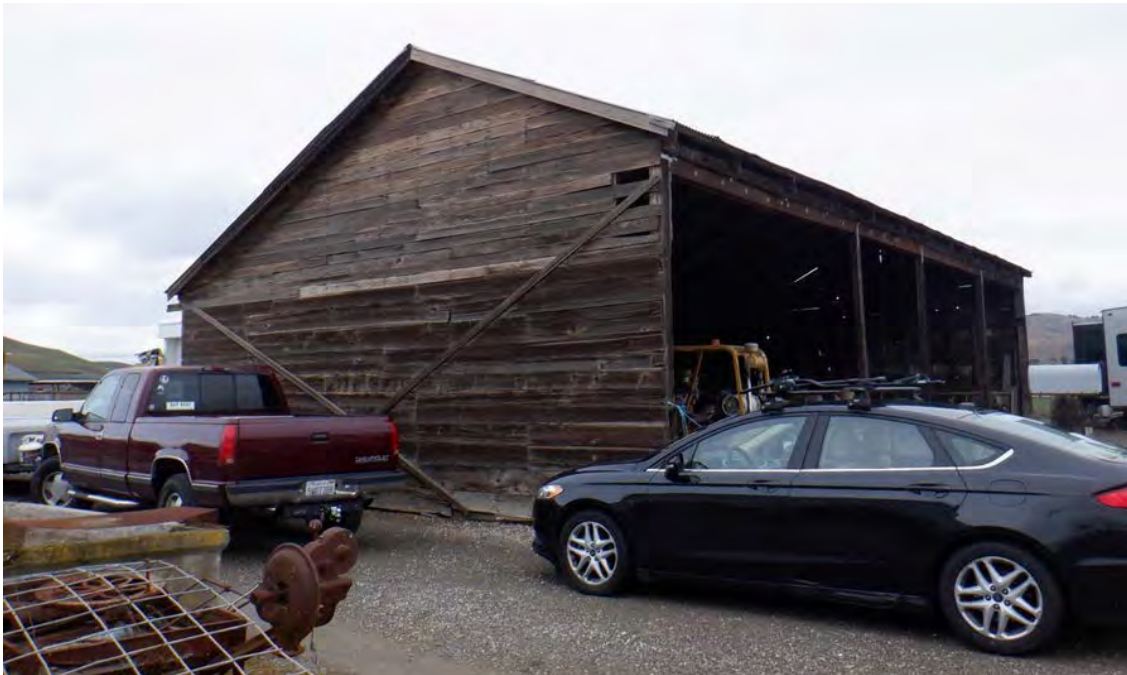
P5b. Description of Photo: Shed south façade with 1"x12" horizontal redwood siding on the lower half and 1"x 6" on the upper half, looking northwest.
