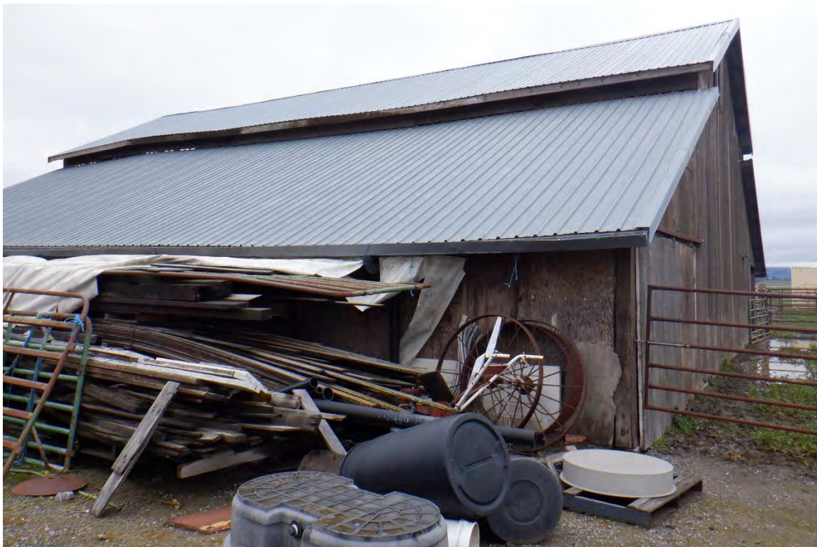
P5b. Description of Photo: Barn north and west façade, looking southeast. Notice the plywood siding on the north façade.
