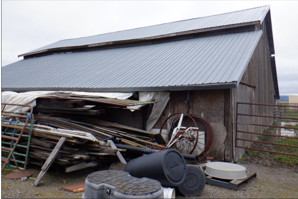
Figure 16. Barn north and west façade, looking southeast. Notice the plywood siding on the north façade
