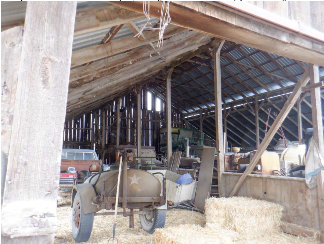
P5b. Description of Photo: Barn interior with post and beam construction and bay dividers, looking west.
