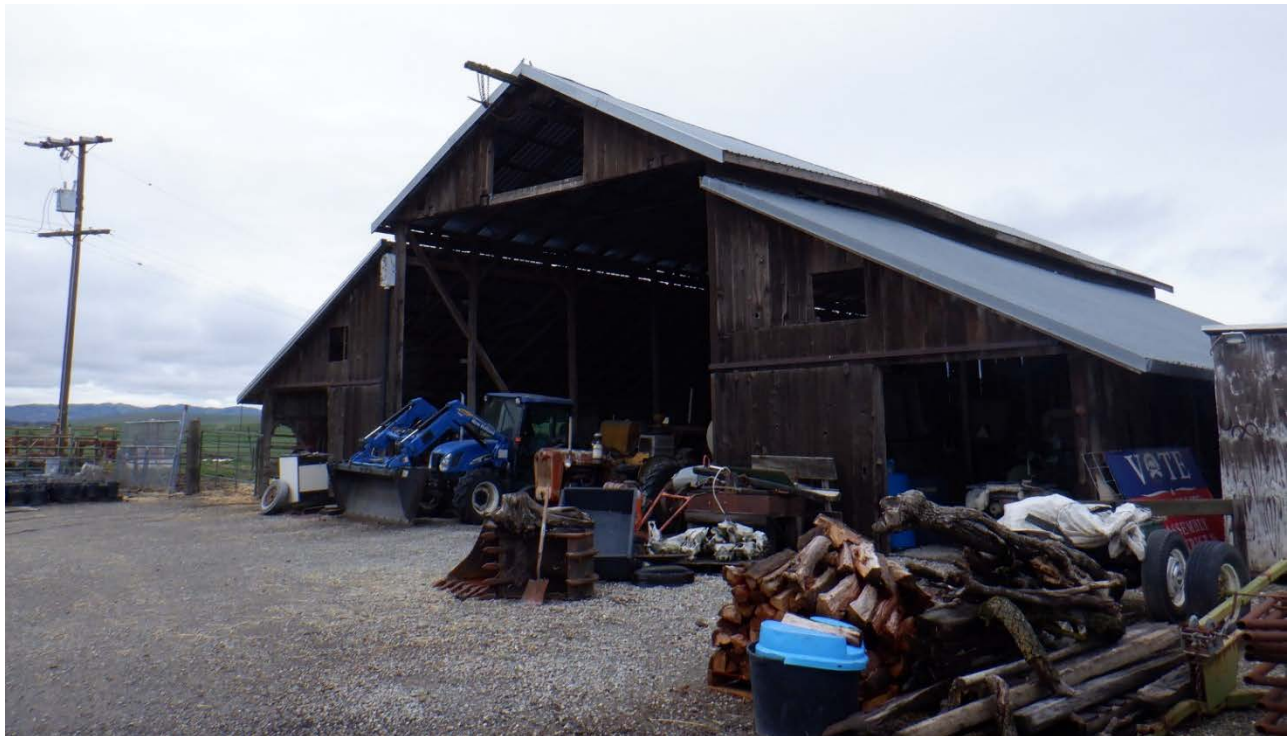
P5b. Description of Photo: Barn east façade, looking southwest. Notice the large expanded opening and the protruding hay rail from the front gable.
