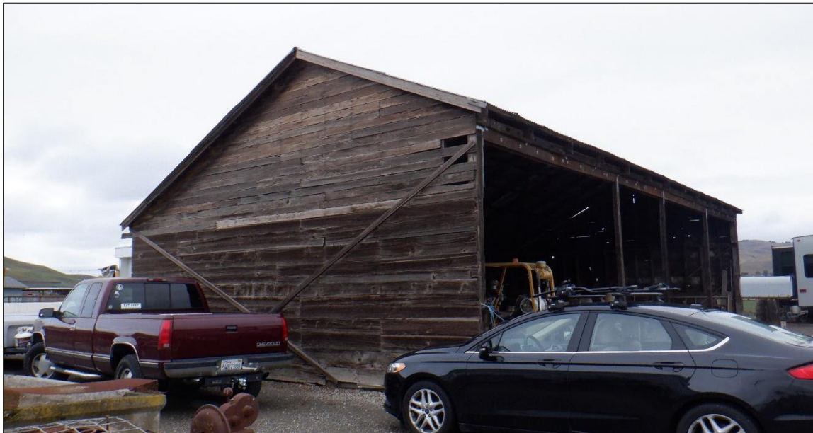
Figure 22. Shed south façade with 1" x 12" horizontal redwood siding on the lower half and 1" x 6" on the upper half, looking northwest
