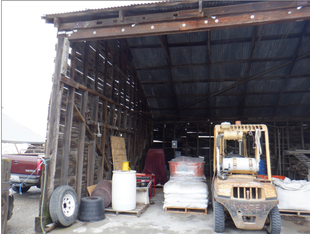
Figure 23. Interior of shed with its post-and-beam construction, looking west. Notice the primary support beam above with metal brackets. An older support beam with mortise rests above the newer primary support beam. This beam most likely comes from an older structure which is a common feature of vernacular ranching structures
