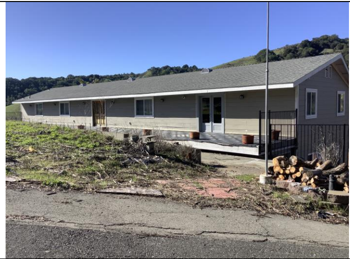
Photo 31. Primary, or east facade and north facade of ancillary residence (Building 4), facing southwest.
