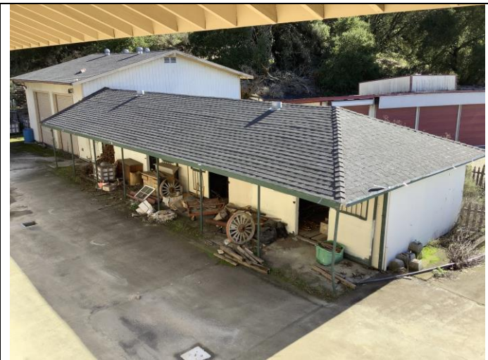
Photo 47. Storage barn with garage addition, facing southwest from upper level of the staircase of open-air garage.
