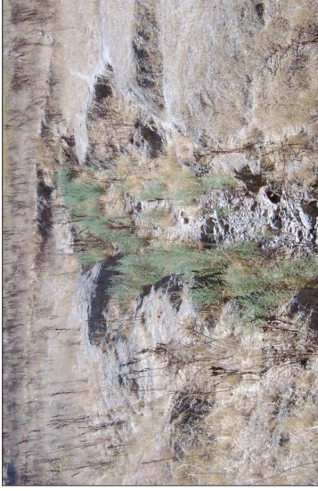
Photo 9: Creek bed erosion
