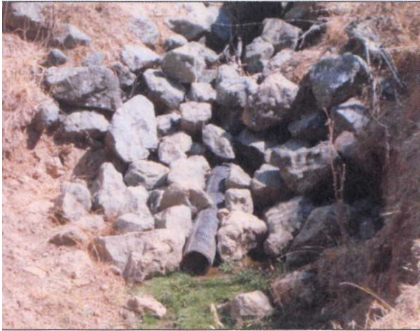
Picture 5: Culvert at the southeastern boundary of the project site where SW 2 receives offsite waters from the adjacent Poppy Ridge Golf Course.
