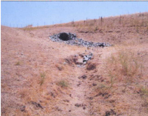
Picture 7: Culvert at the southern end of the project site where ED 5 originates.
