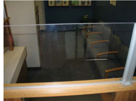
Inadequate public counter at the Coroner's Building
