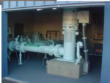
Emergency Well and Pump
