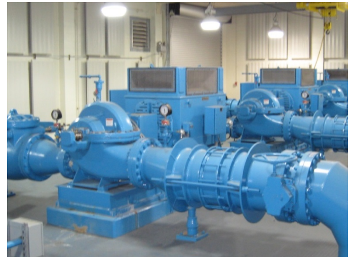
Hesperian Pump Station
