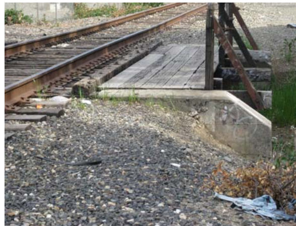
Multi-use pathway alignments along the Oakland Subdivision require grade-separation of many small drainage features.
